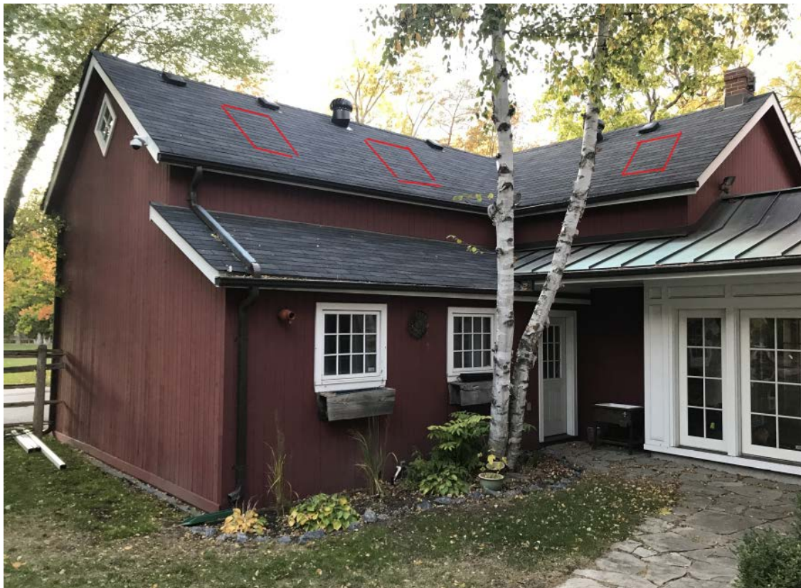
Proposed skylights on rear roof slopes of barn, out of street view.
