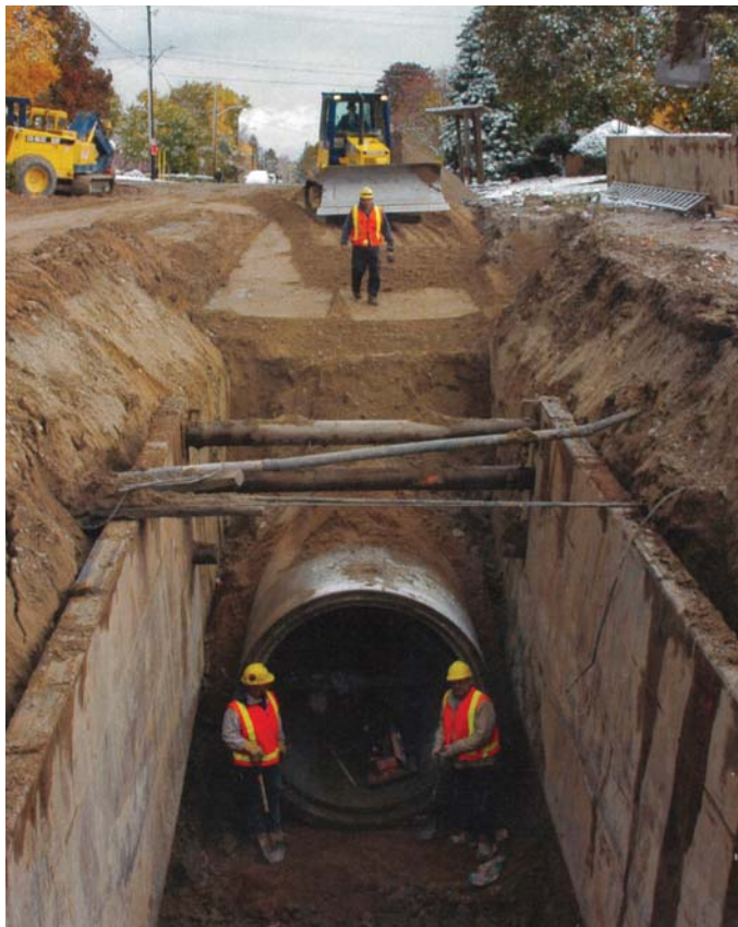
Installation of a new stormwater pipe as part of the Markham Flood Control Program.
