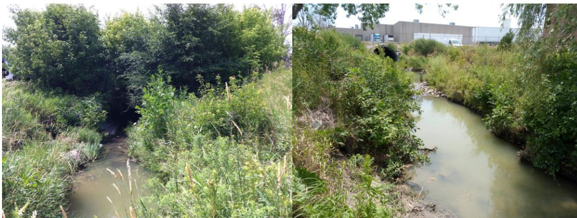
Culvert Inlet – Note slope failure on left side of inlet Culvert outlet and restoration works at 300 Steelcase Rd
