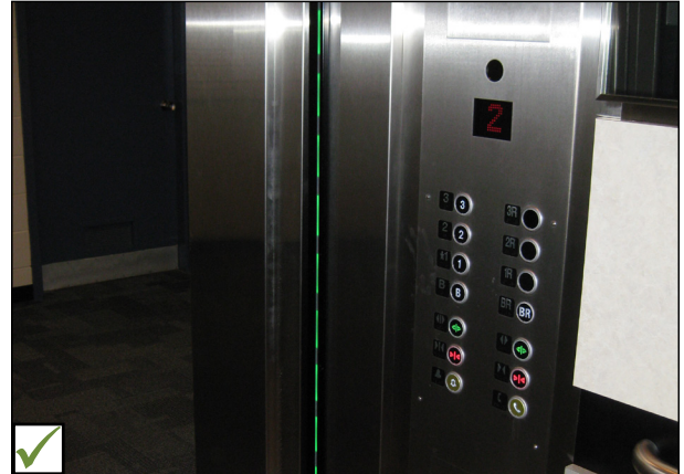
Elevator sensor door and floor registration buttons.
