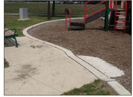
Curb ramp into play space where there is a level change between accessible route and play space.
