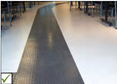
Tactile floor surface to guide users with vision loss.
