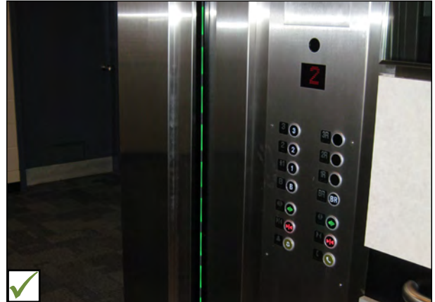
Elevator sensor door and floor registration buttons.
