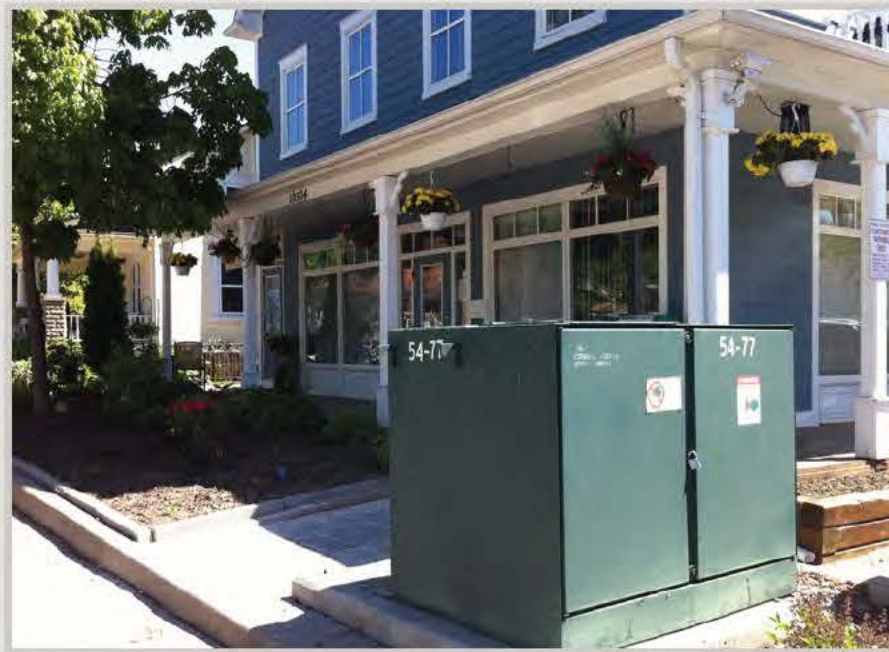
Throughout the village, externalized utility boxes are located in the sidewalk area interrupting the pedestrian streetscape
