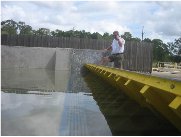
Flood gate operating during flooding conditions (source: floodbreak.com )
