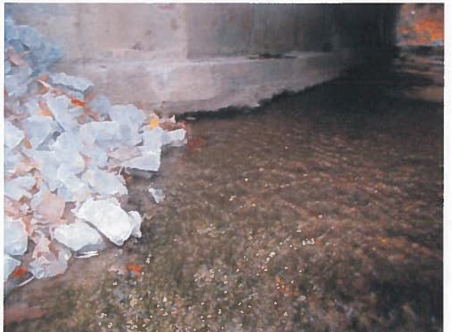
Bridge pier undercutting - East Don River Tributary
