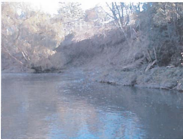
Erosion in private yards - Rouge River
