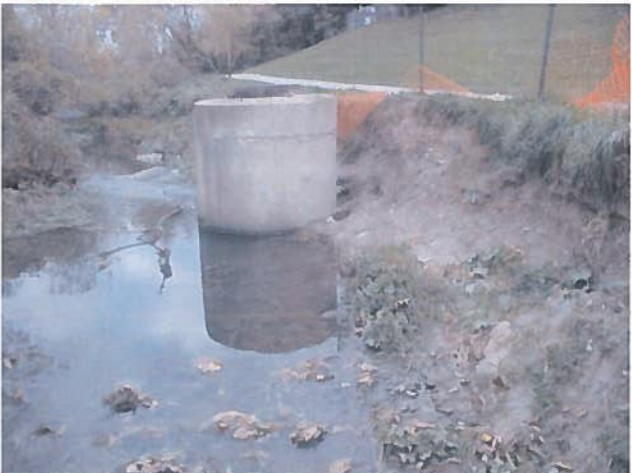
Exposed Manhole - Mt. Joy Creek
