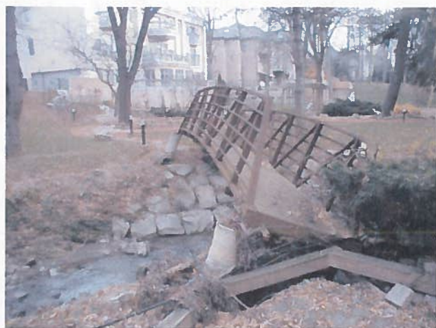
Bridge failure - East Don River Tributary
