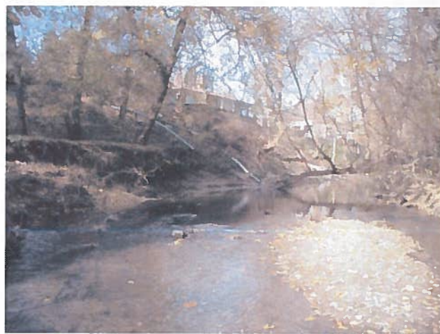
Erosion in private yards - East Don River
