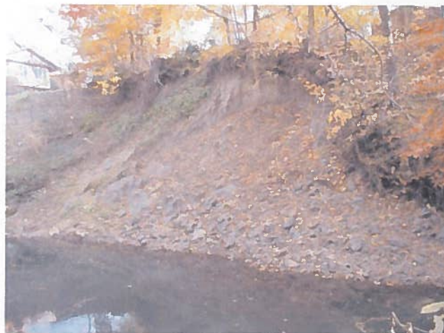
Valley wall erosion - East Don River
