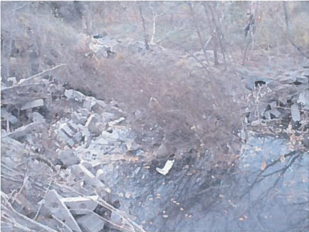
Upheaval of existing bed protection - German Mills Creek Tributary
