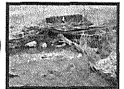
Culvert Blocked with Debris
