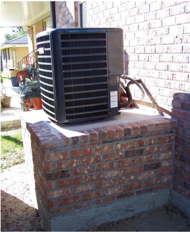
Air conditioning / heat pump compressor mounted on a brick pedestal above the High Water Level (source: fema.gov )
