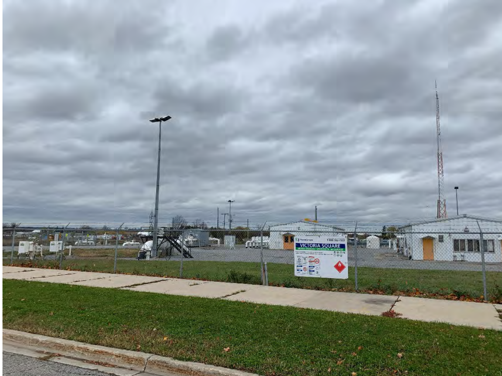
Photo 15: View towards the east of the TransCanada Victoria Square (natural gas) meter station 11346 Woodbine Avenue.
